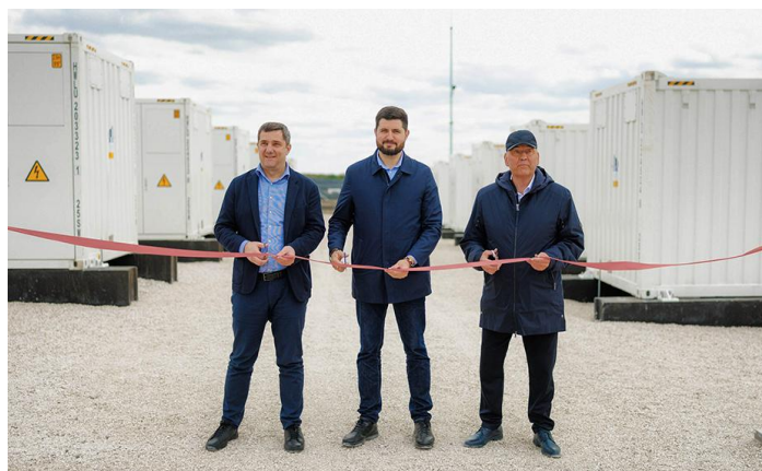
Maib financed the construction of a 60 MWh battery energy storage system (BESS)
